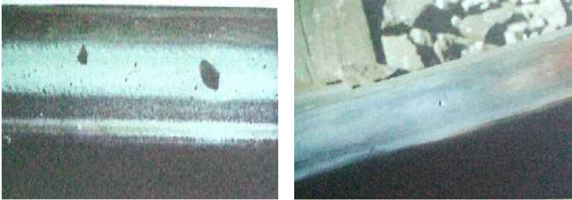
FIG. 48 : 301 - DAMAGE TO RAIL BY BRUSHING OR ARCING
